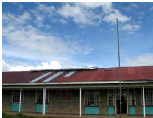
Secondary school with PV system
