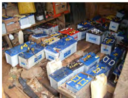
Inside the charging shop
