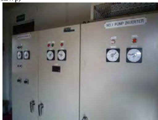
Control panel and inverter
