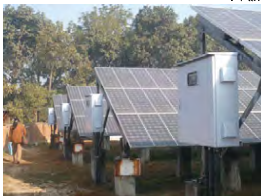
PV sub-array and connection box
