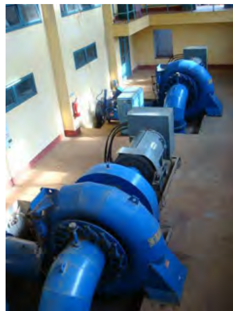
Photograph 51-2 Inside of O'Chum 2 Powerhouse
