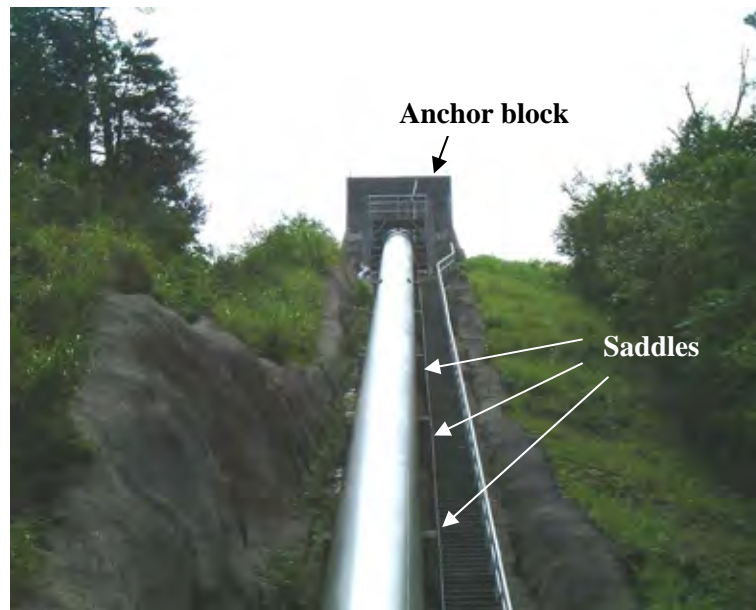
Photograph 48-3 Penstock, Anchor Block and Saddles
