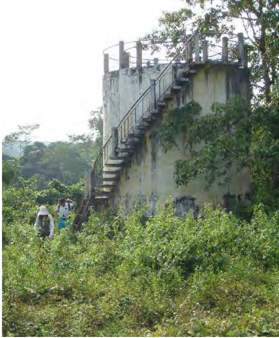
Photograph 47-1 Sample of Surge Tank
