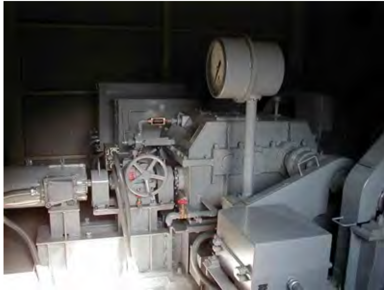
Photograph 50-6 Hoist of Intake Gate
