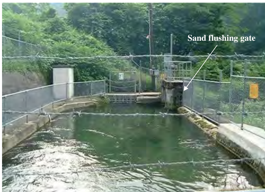
Photograph 44-2 Settling Basin of the Other Station
