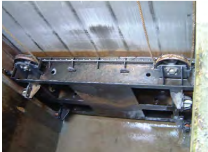
Photograph 50-4 Fixed Wheel Gate
