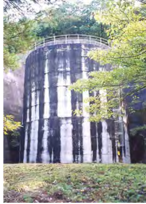
Photograph 47-2 Sample of Surge Tank
