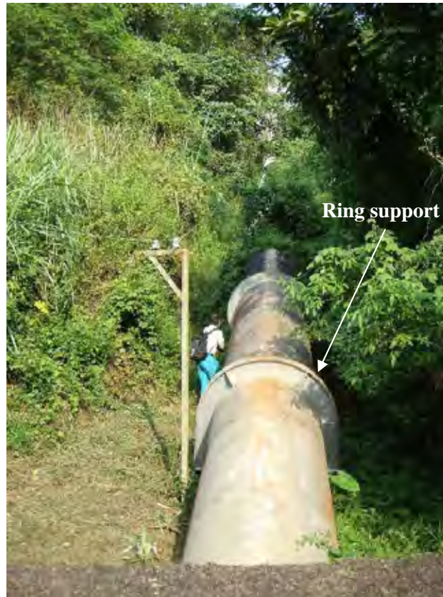
Photograph 48-1 Penstock of O'Chum 2 Hydropower Station
