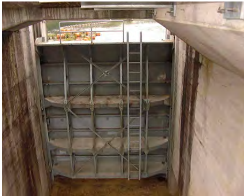
Photograph 50-2 Fixed Wheel Gate
