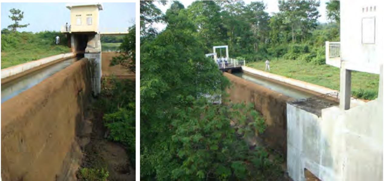
Photograph 44-1 Settling Basin of the O'Chum 2 Hydropower Station
