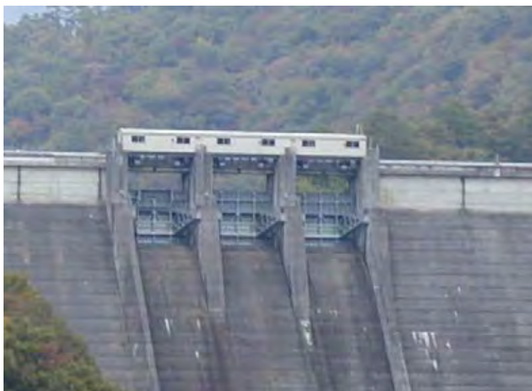
Photograph 40-1 Spillway Gate (Radial Gate) and Hoist
