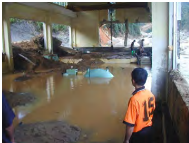
Photograph 18-1 Flooded Powerhouse (Nam Phao Hydropower Station Case in Lao PDR)
