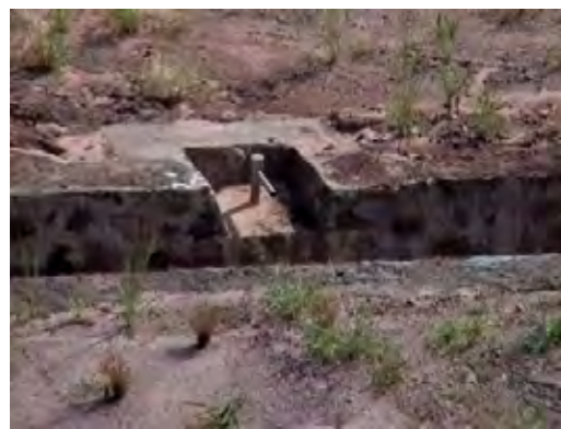
Photograph 26-2 Instrument for Monitoring Seepage
