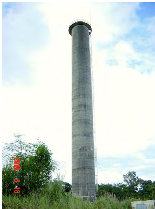
Photo 5.3-5 Tower Type Surge Tank, Kirirom 1 Hydropower Station (photo as of August 16, 2004)
