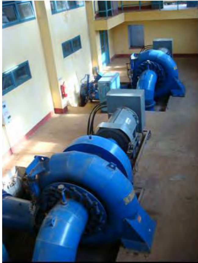
Photo 5.2-6 Turbine and Generator of O’chum 2 Hydropower Station
