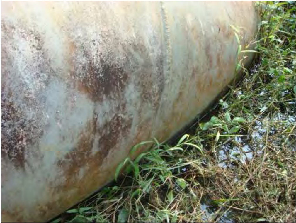
Photo 5.2-8 Junction of Penstock and Lower end Anchor Block of O’chum 2 Power Station
