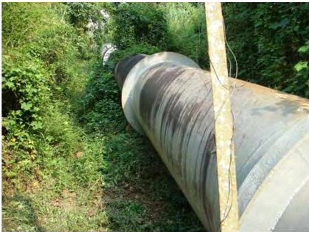
Photo 5.2-7 Penstock of O’chum 2 Hydropower Station
