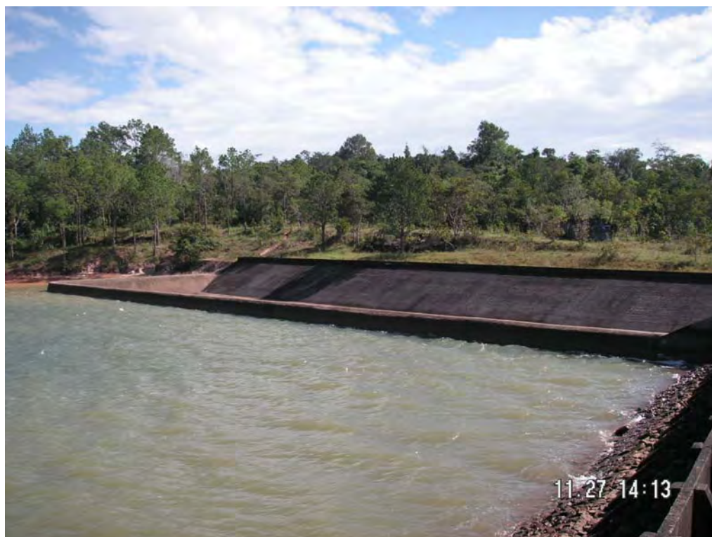
Photo 5.3-3 Lateral Overflow Weir of Gateless Type Service Spillway at Left Abutment of Dam, Kirirom 1 Hydropower Station
