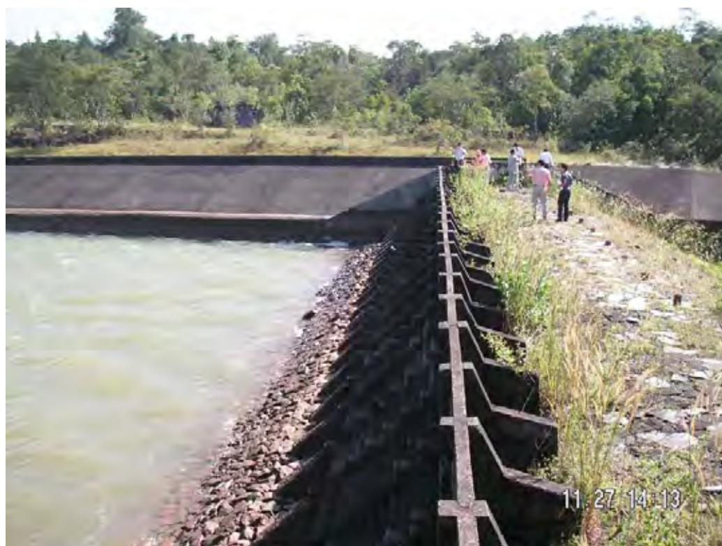
Photo 5.3-4 Fuse Plug Type Emergency Spillway at Left Abutment of Dam, Kirirom 1 Hydropower Station
