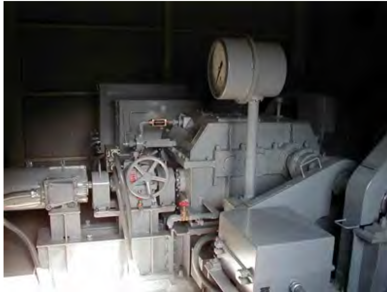
Photograph 50-6 Hoist of Intake Gate
