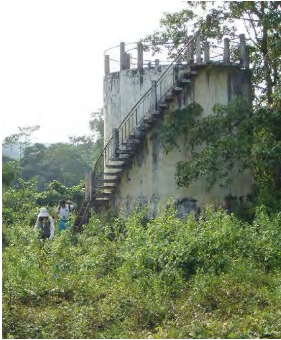
Photograph 47-1 Sample of Surge Tank
