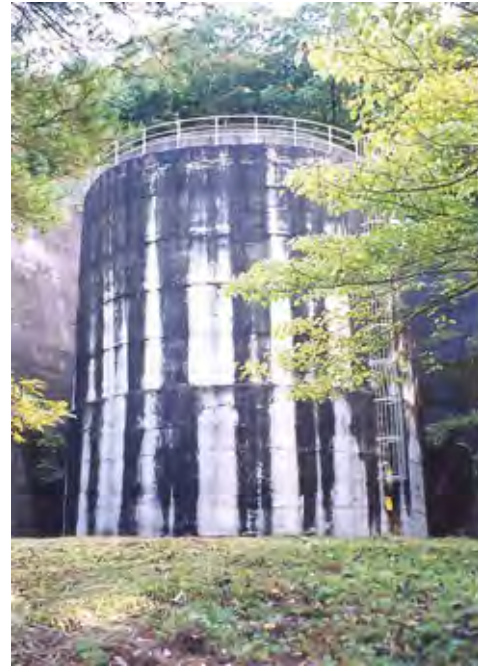
Photograph 47-2 Sample of Surge Tank
