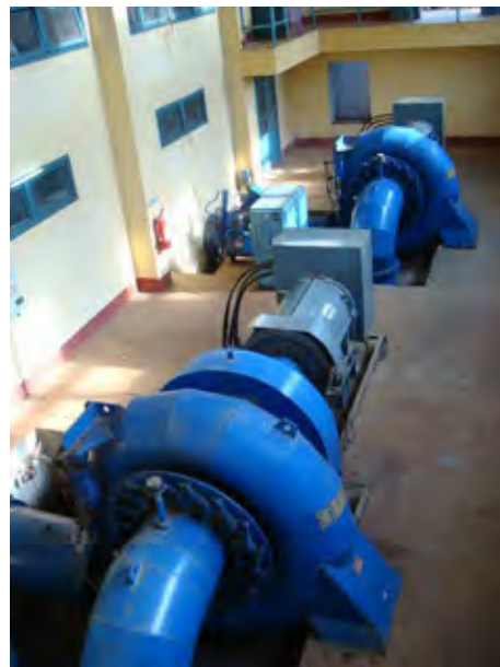
Photograph 51-2 Inside of O'Chum 2 Powerhouse
