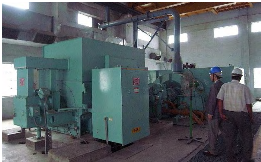
Picture 3-B Cement Kiln Waste Heat Recovery System Generator
