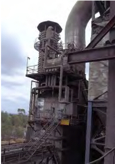
Picture 3-A Cement Kiln Waste Heat Recovery System
