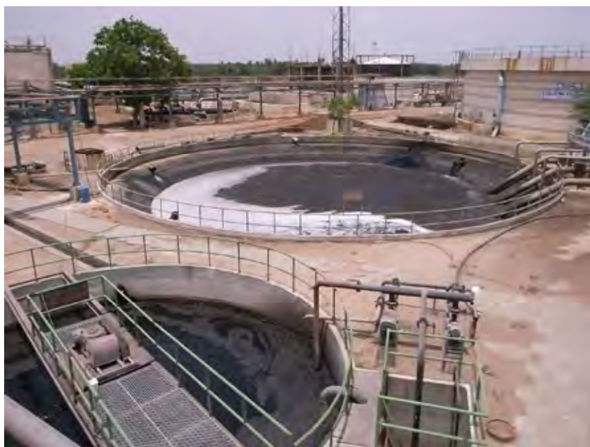
Picture 7-E Waste Water Treatment Facility
