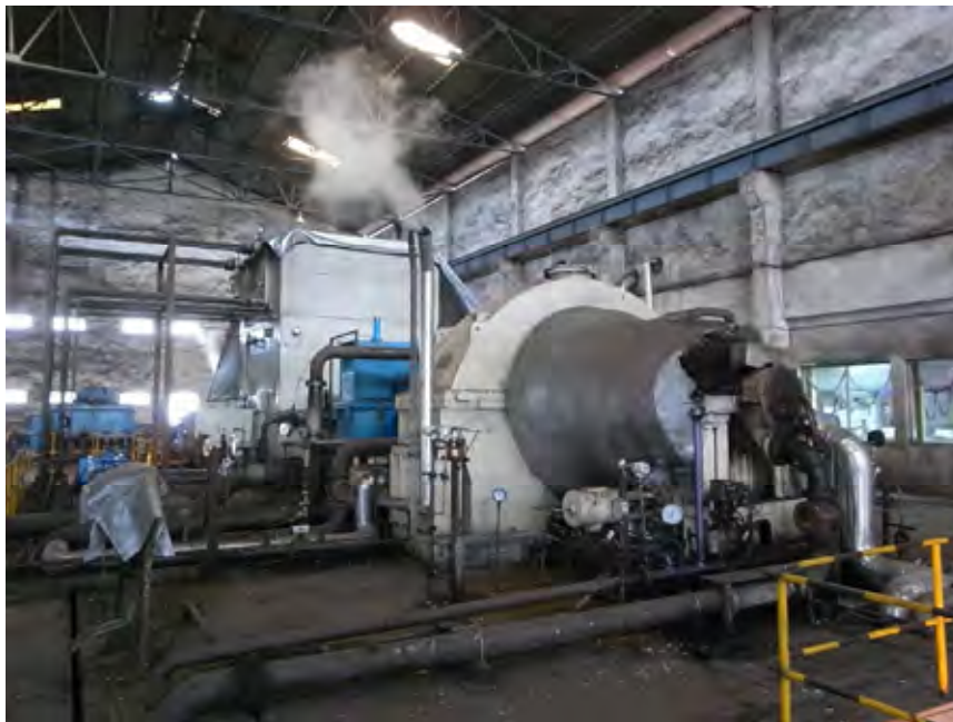
Picture 7-B Waste Heat Recovery System (Steam turbine power generator)
