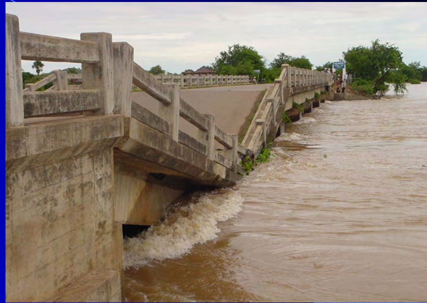
Bridge on the National Road 6A was collapsed by year 2001 Mekong River Flood, in Kompong Cham Province
