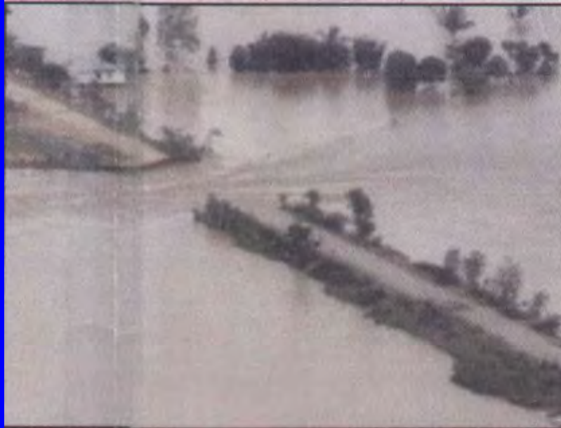
Collapse of embankment of national road No 1 by overland flow from right bank side of Mekong river during the flood in year 2000
