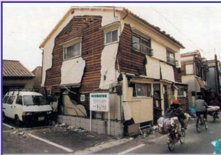
(Damage to the wall)
