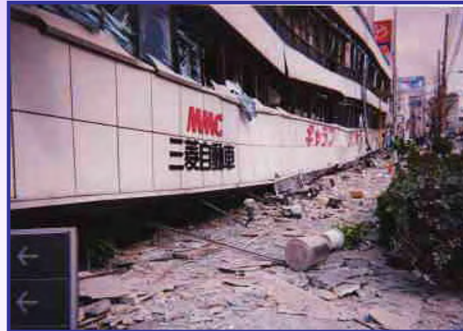
(Collapse of the 1 st floor)
