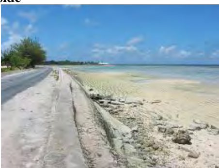
Photo 3 Damage to the causeway revetment
