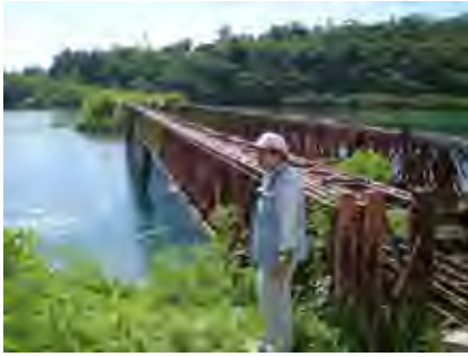
Full view of bridge (prohibited passage)
