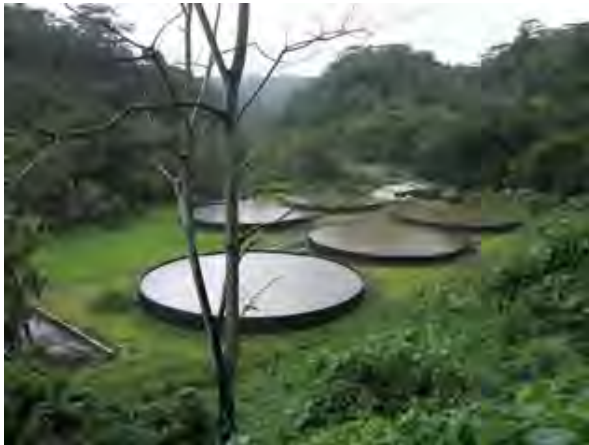
Slow filtration facilities
