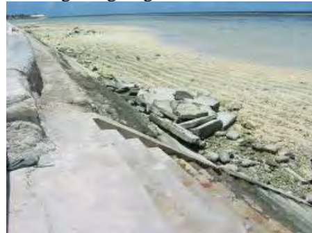
Photo 2 Damage to the causeway revetment
