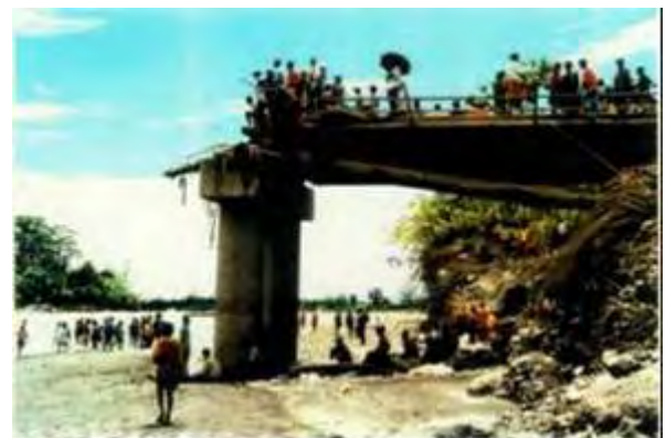
Photo 2-2.8 Bridge Damage Caused by the Boana Flood (Provided by the Geological Survey Office)
