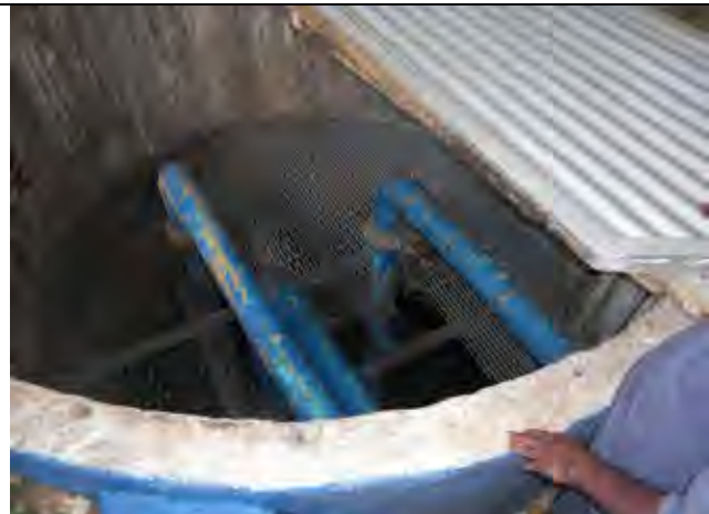
Shallow well for water supply source (Luganville-Vanuatu). It is located where the well might be submerged in torrential rainfall.
