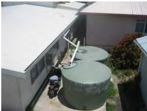
Rainwater storage tank
