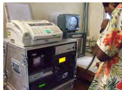
Photo 2-2.11 Transmitter/Receiver at an Observation Center
