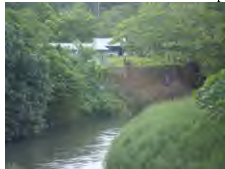
Bank slip upstream of the bridge (The houses nearby are in a dangerous position)
