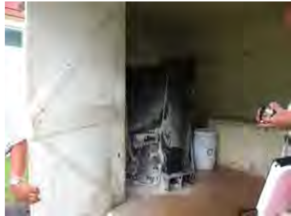
Chlorine injection equipment
