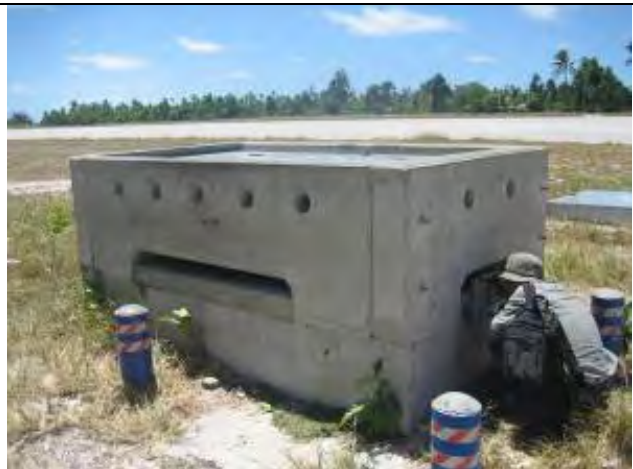
A well for public water supply in Tarawa of Kiribati. Salinization of groundwater of this well is advancing and new groundwater development is planned.
