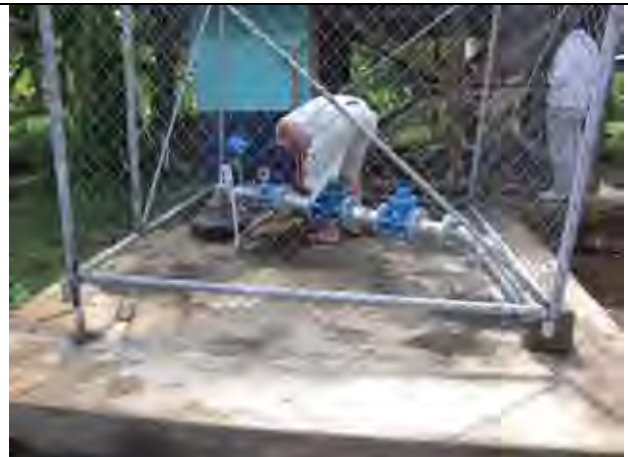
Facilities for rural water supply managed by the Government (Luhiluhi village in Samoa). Government is shifting water sources from springs and shallow wells with water quality problems to safety sources of the Government.
