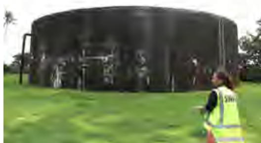
Distribution reservoir (capacity 2,500m 3 )
