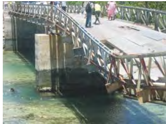
Photo 2-2.4 Damaged Water Pipe on the Side of the Bridge
