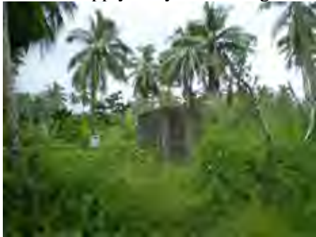
Water supply tank in Utulei Village
