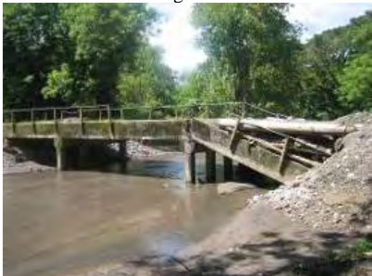
Bridge with collapsed connection
