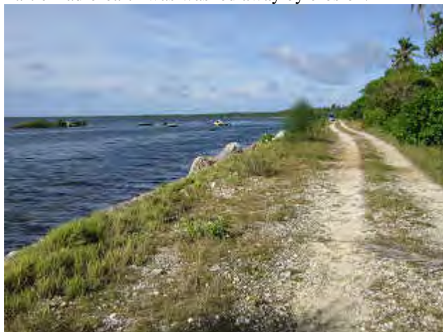
The previous shoreline is seen in left side of this photo. Seawall was newly constructed by support of Canada, but seawall is inundated by overtopping of waves when cyclone.
