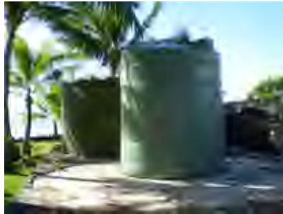
Hotel water supply tanks (made in Samoa)
