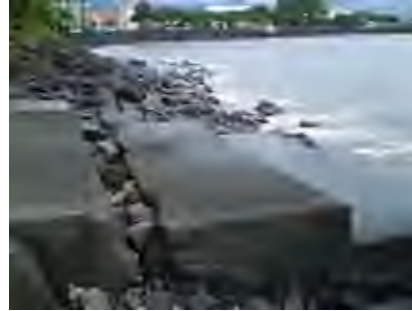
Revetment damage caused by high tides
