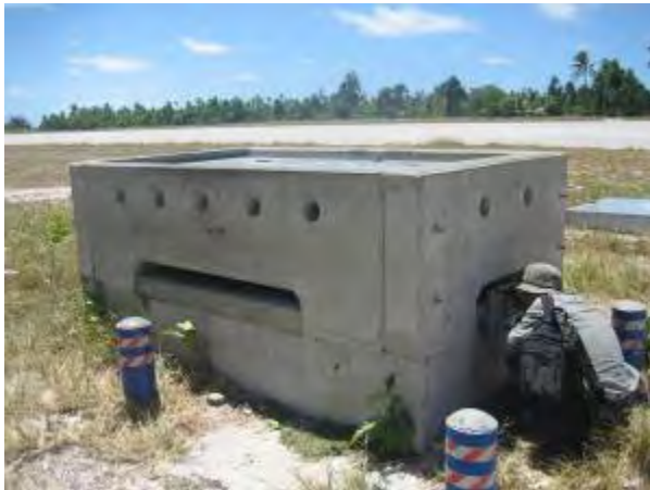
Photo 11 Government water supply source (wells) – installed near the airfield
