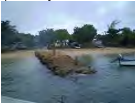
Existing jetty (extreme deterioration)
