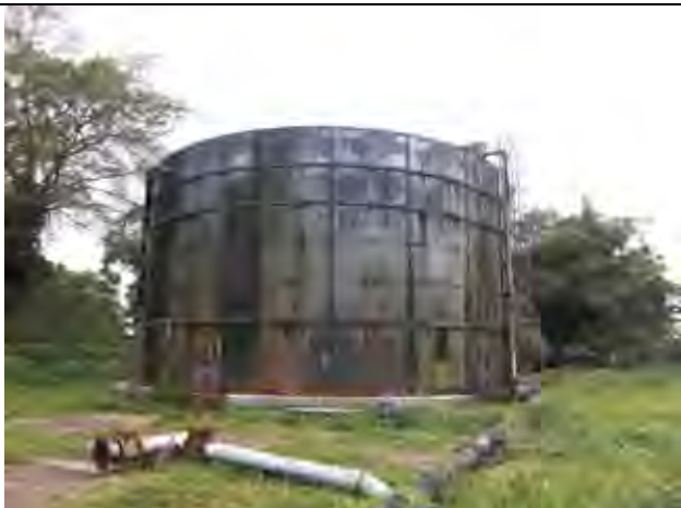
Distribution reservoir made of steel (Luganville-Vanuatu). This tank is too old to distribute water in emergency.
