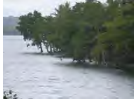
Rising sea level downstream of Sarakata Bridge (Scouring has occurred around tree roots)
