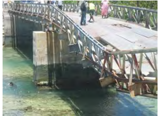
Photo 10 Damage to the bridge linking Tanaea and Buota districts
