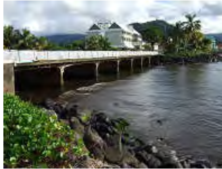
The Beach Road bridge at the river mouth. Low-lying land at and upstream of the bridge was inundated. The coastal side is protected by a solid stone seawall.
