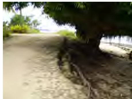
High tides have caused erosion of roads
