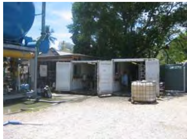
Seawater desalination plant
