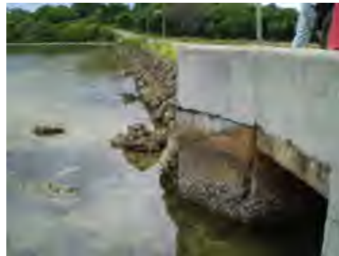
Corrosion of the box culvert (Seawater rises to the top of the box culvert)
