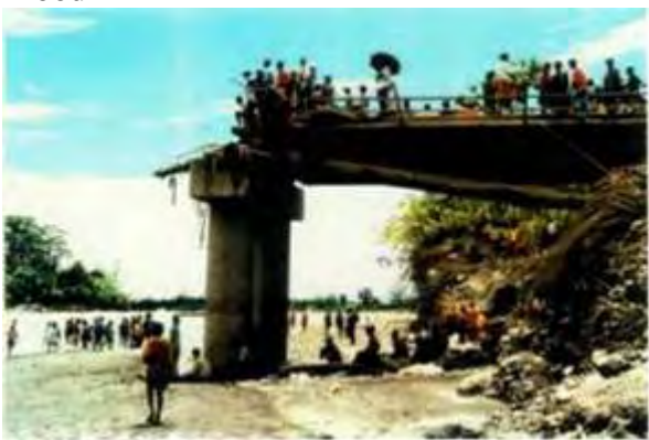
Damage of road bridge by Boana flood in Pupa new guinea (NDC). Trunk road in local area was interrupted and big damage was given to daily life in rural residents.
