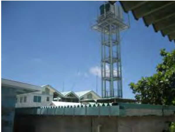
Photo 9 Storage tank and elevated tank at Tungaru Central Hospital
