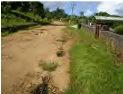
Poor road drainage conditions and damaged road surface
