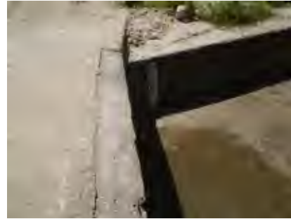
Sediment accumulation can be seen upstream (Ditto)
