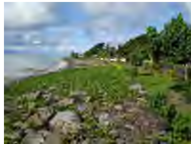
Stone masonry seawall (Gentle slope in line with the coastal terrain and built higher than the road surface)
