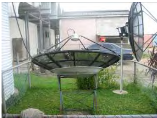
Satellite receiving equipment
