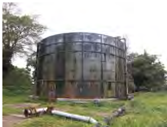
Distribution reservoir (capacity 1,100m 3 )
