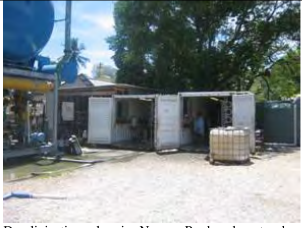
Desalinization plant in Nauru. Produced water by the plants is only drinkable water in dry season. They have only 3 water trucks and water delivery is usually delayed.
