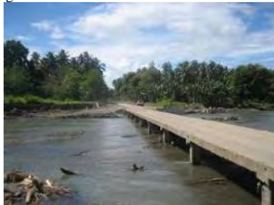
Vmasni River where the area around the connection on the right bank has been eroded
