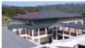
Roof of a gymnasium (inside the red line is 10 kW PV modules)
