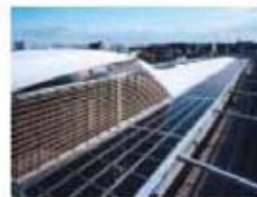
Roof of a station (140 kW see-through type PV modules)
