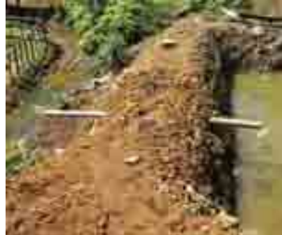
Overflow (outlet) pipe
