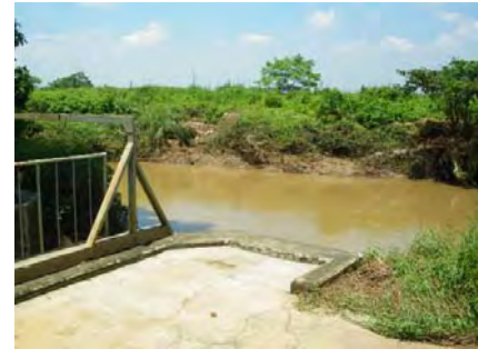
Figure 2.1.35 Raw Water Intake
