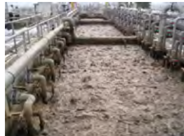
Figure 3.1.28 MBR Reactor Tank
