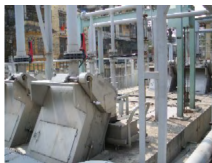
Figure 3.1.10 Odor Plumbing of Screen Facility
