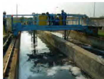
Figure 3.1.25 Grit Chamber and Inspection
