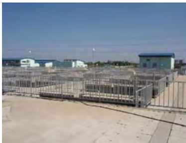
Figure 3.1.15 Binh Hung WWTP
