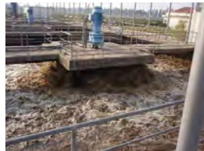
Figure 3.1.4 Aerator of North Thang Long WWTP
