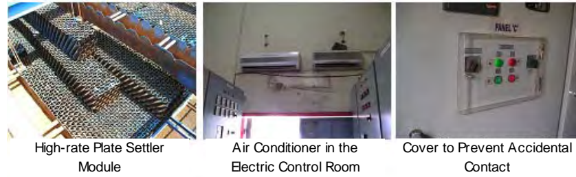
Figure 2.1.30 Example of Devices on O&M in Cikokol Purification Plant
