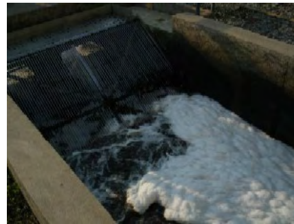
Figure 3.1.22 Inlet and Screenings
