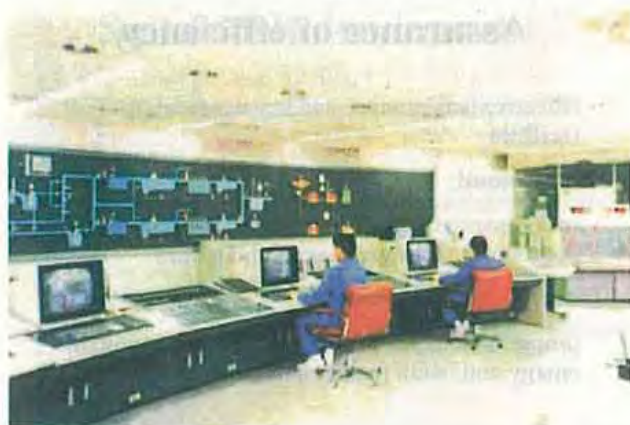
Wastewater treatment plant control room
