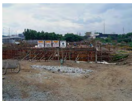
Photo 4.3.2: Ongoing construction works for the 10,000 m 3 /day Olandes Sewage Treatment Plant along the Marikina River. The project is one of the components of the MTSP.
