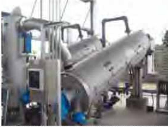
Photo 2.3.9: Screw press equipment used to dewater sludge at the MWCI San Mateo (South) septage treatment plant. This type of equipment is also used at the MWCI North and MWSI Dagat-Dagatan septage treatment plants.
