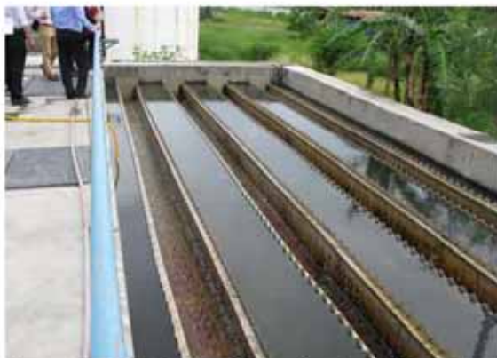
Photo 2.3.5: Sedimentation tank at the Global City STP operated by MWCI
