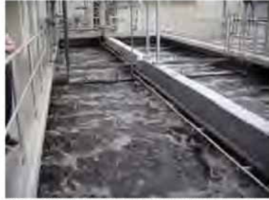
Photo 2.3.10: Aeration tanks (activated sludge process) used for treating filtrate coming from the screw presses.
