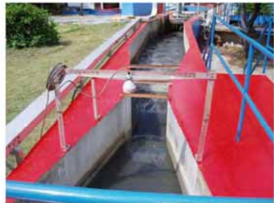
Photo 2.3.4: Mechanical screening facility
