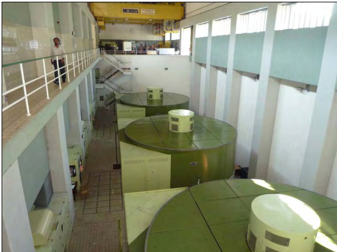
Existing Powerhouse Units
