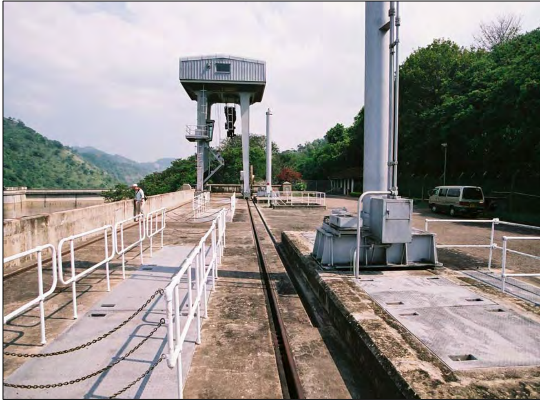
Existing Intake for Expansion
