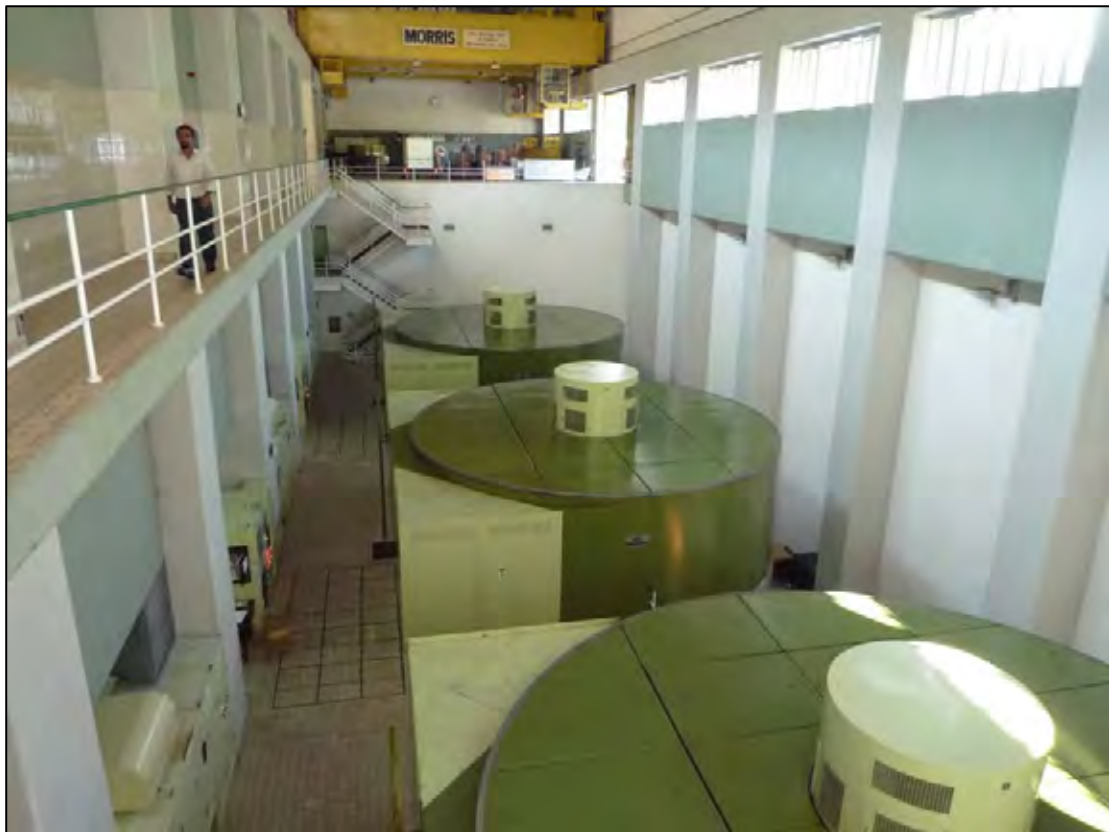
Existing Powerhouse Units
