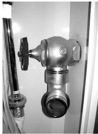
Photo. 40.12 An example of a water discharge outlet mounted on a fire hydrant box
