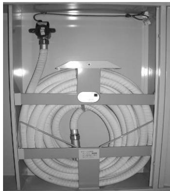
Photo. 40.8 Easy-to-handle-type No. 1 fire hydrant
