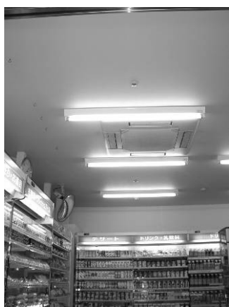
Photo 40.11 An example of a sprinkler installed in a convenience-store-type stand
