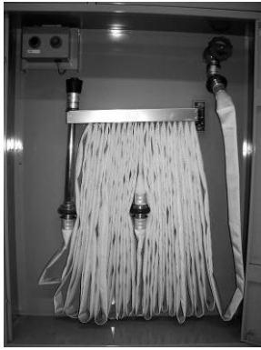
Photo. 40.7 An example of the No.1 fire hydrant
