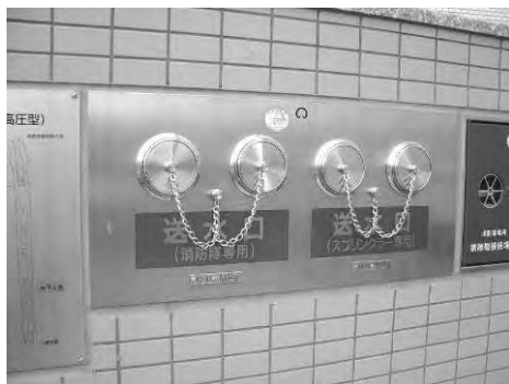
Photo. 40.13 An example of water supply outlets mounted at an entrance
