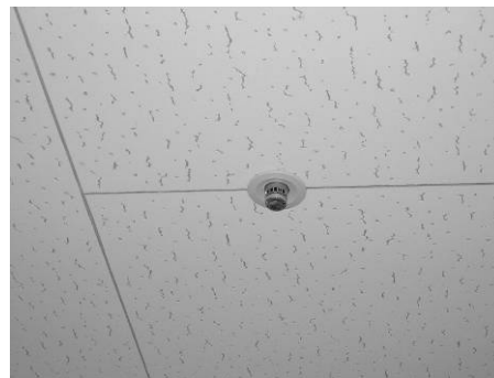
Photo. 40.10 An example of sprinkler heads
