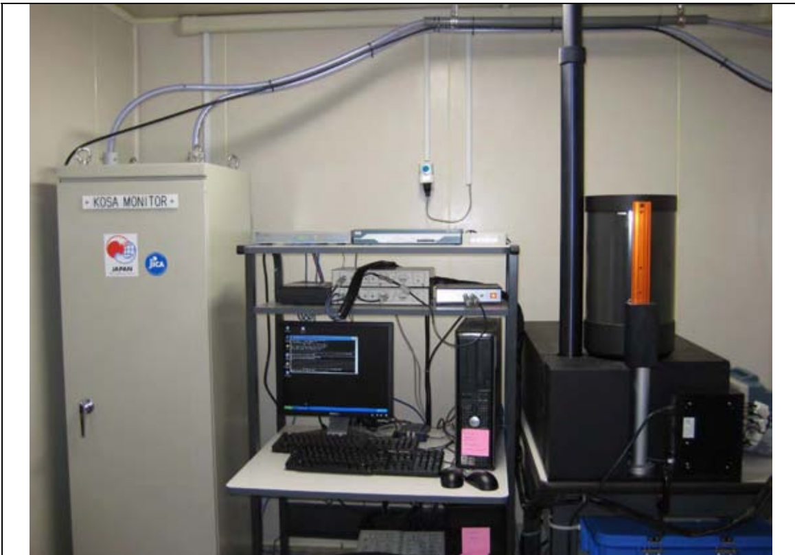
Zamin-ud Meteorological Station (Equipment installed in the Container) 18 August, 2007
