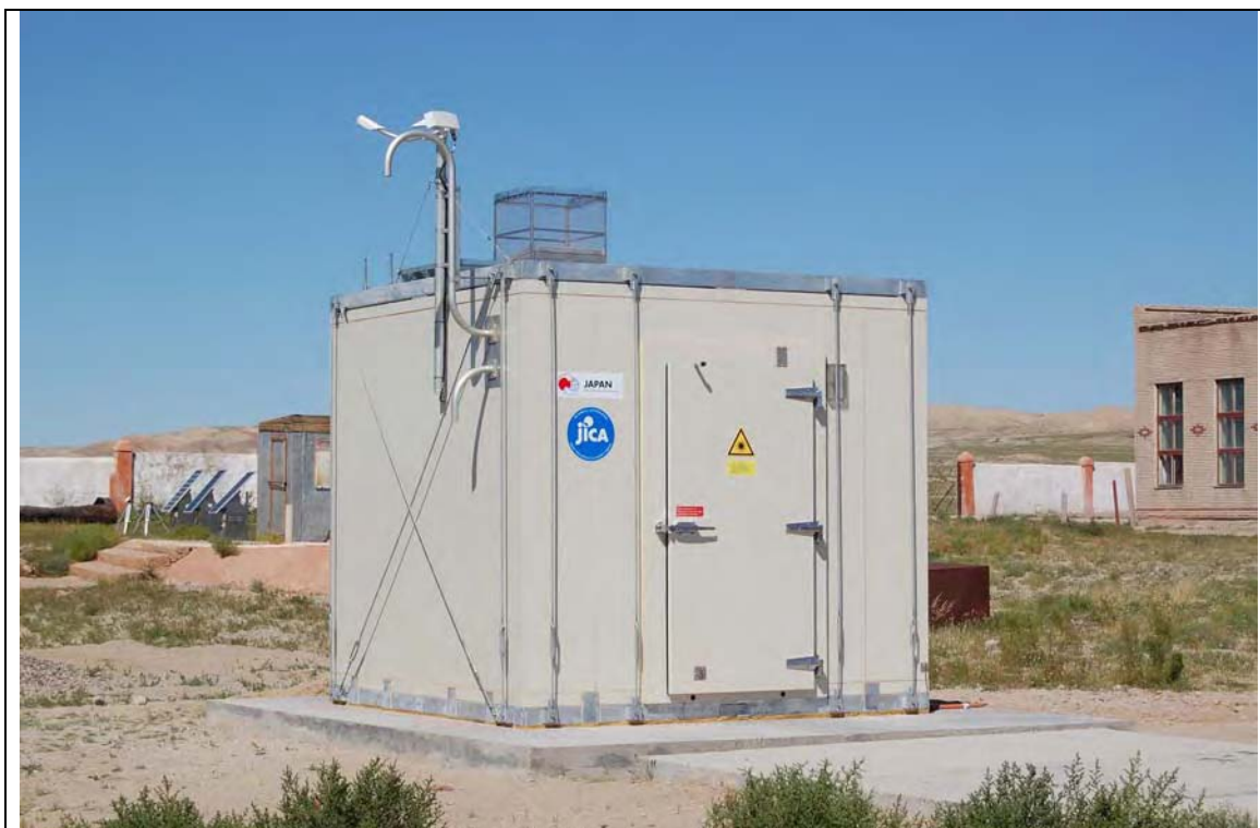
Completion of the Equipment Installation Work at Sain Shand Aimag Center 25 August, 2007
