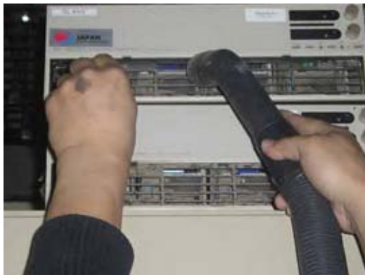
Cleaning Focus Coil Power Supply
