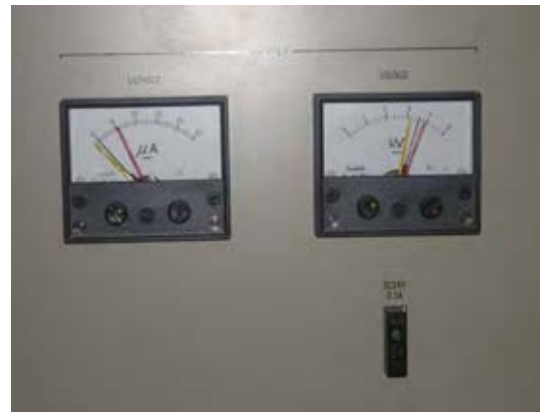
Meter of Ion PUMP PS
