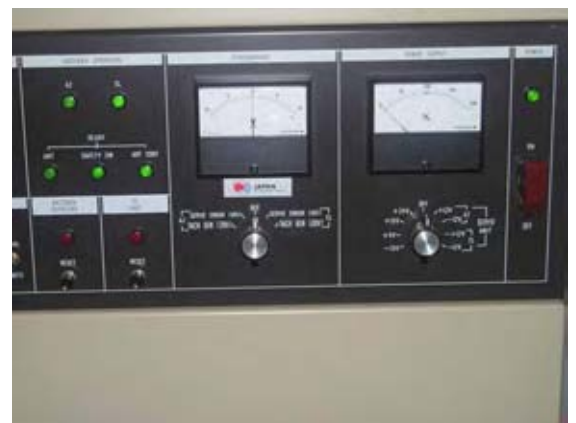
Meter on AVC Operation Panel of AVC
