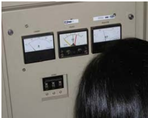
Meters on HV PS 2 panel
