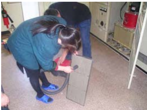
Cleaning of air filter
