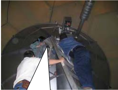
Check the Antenna positioning accuracy by rotating the gears in the azimuth direction
