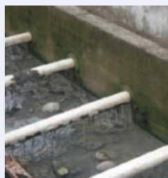
Sewage pipe in Panama Metropolitan area
