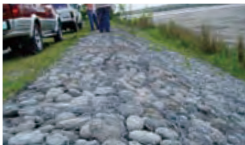
Rehabilitation of a levee on the right bank of the Tarlac River
