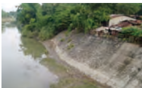
Bank revetment along the Sinocalan River
