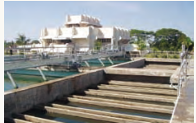
Water supply project in Batangas City in the Philippines: Water Treatment Plant, precipitation system
