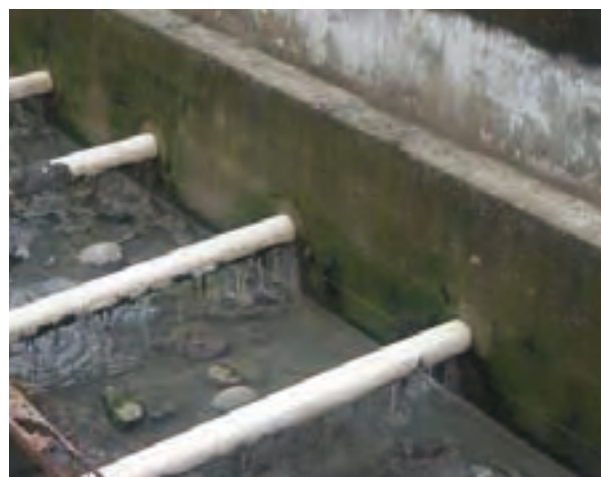
Sewage pipe in Panama Metropolitan area
