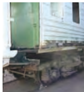
Carriage with peeling paint prior to repair work.
