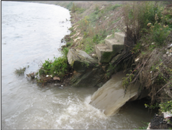
Point (C) Keramidnica (Outlet of Sewerage, Left Bank)
