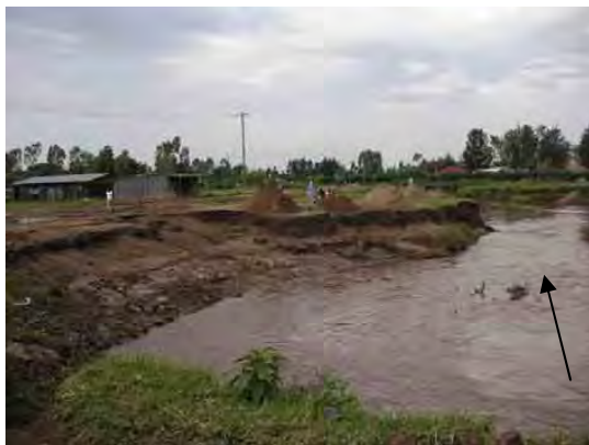
Eroded Riverbank in Nyamasaria River
