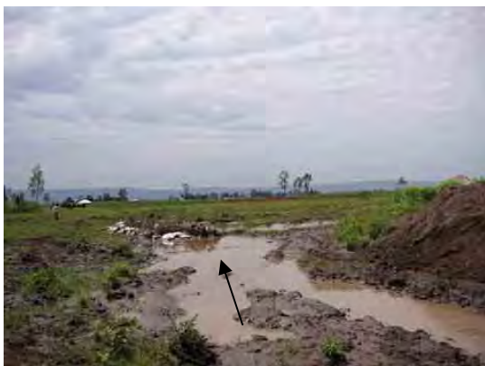
Damaged Dyke on Right Bank
