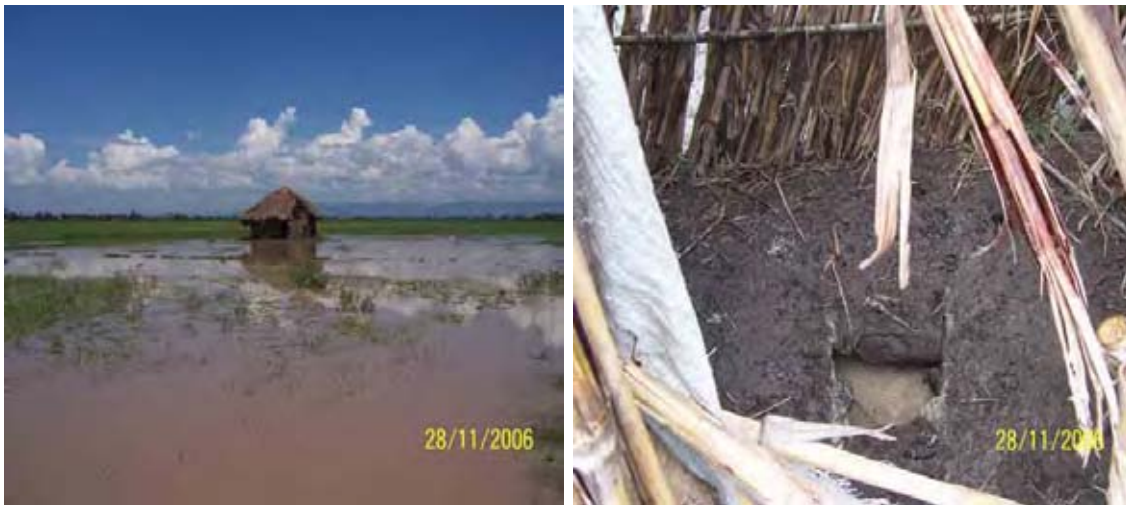
Plate 9&10: Collapsed building after floods (left) and latrine (right)
