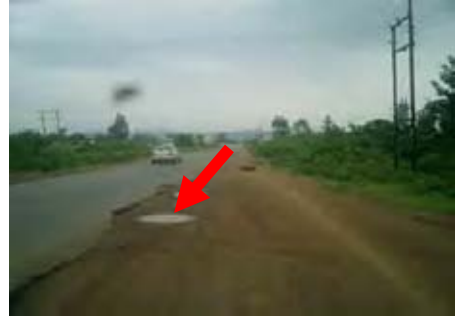
Plate 8: Destroyed road with pothole
