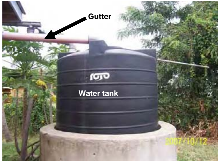
Plate 9: The Water tank for roof water harvesting
