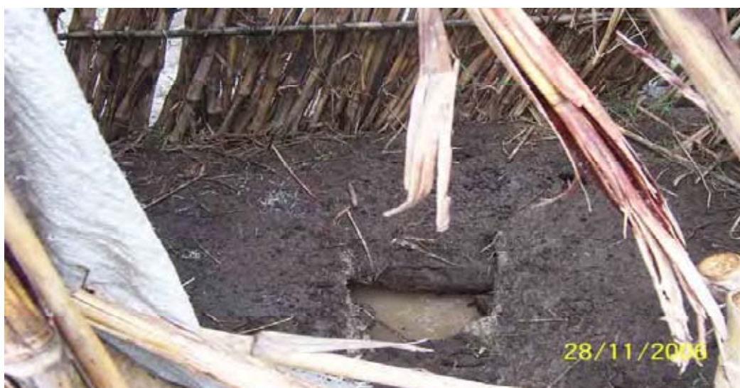
Plate 22 Collapsed latrine after Flood
