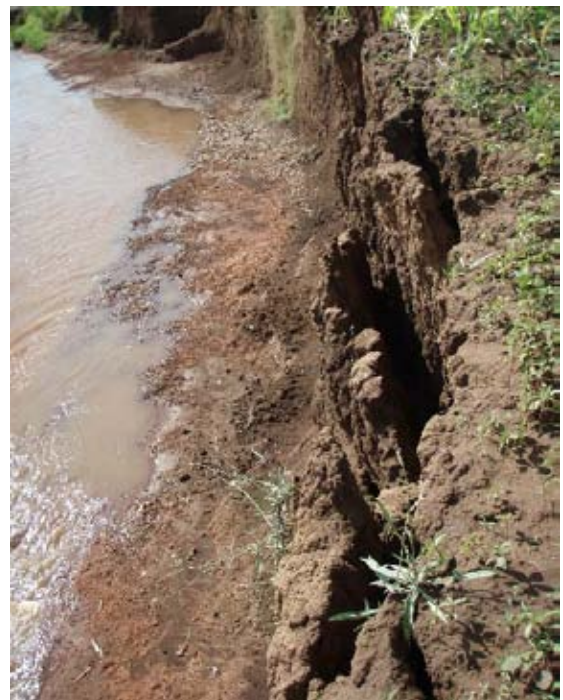
Plate 6 Cracks at River Bank
