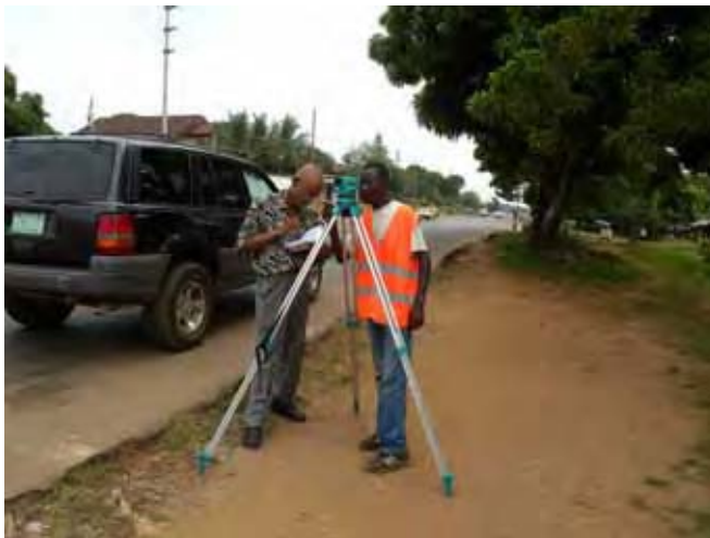
*Left photograph shows simple leveling work with the help of LCS guide.
