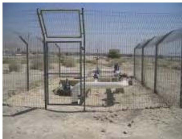
Photo: Connection Point of Mekorot Pipeline (as of July 2008)
