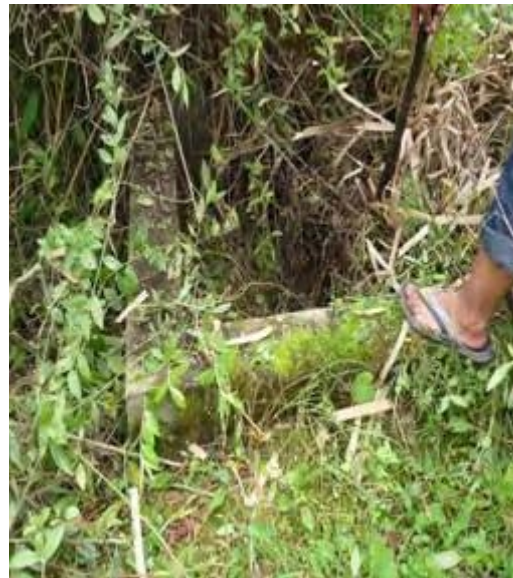
Inter connection Structure
