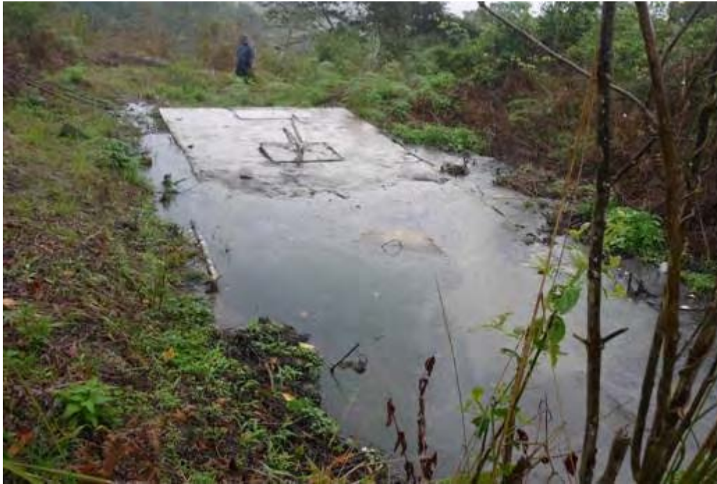
Sewage treatment – Flooded Septic Tank
