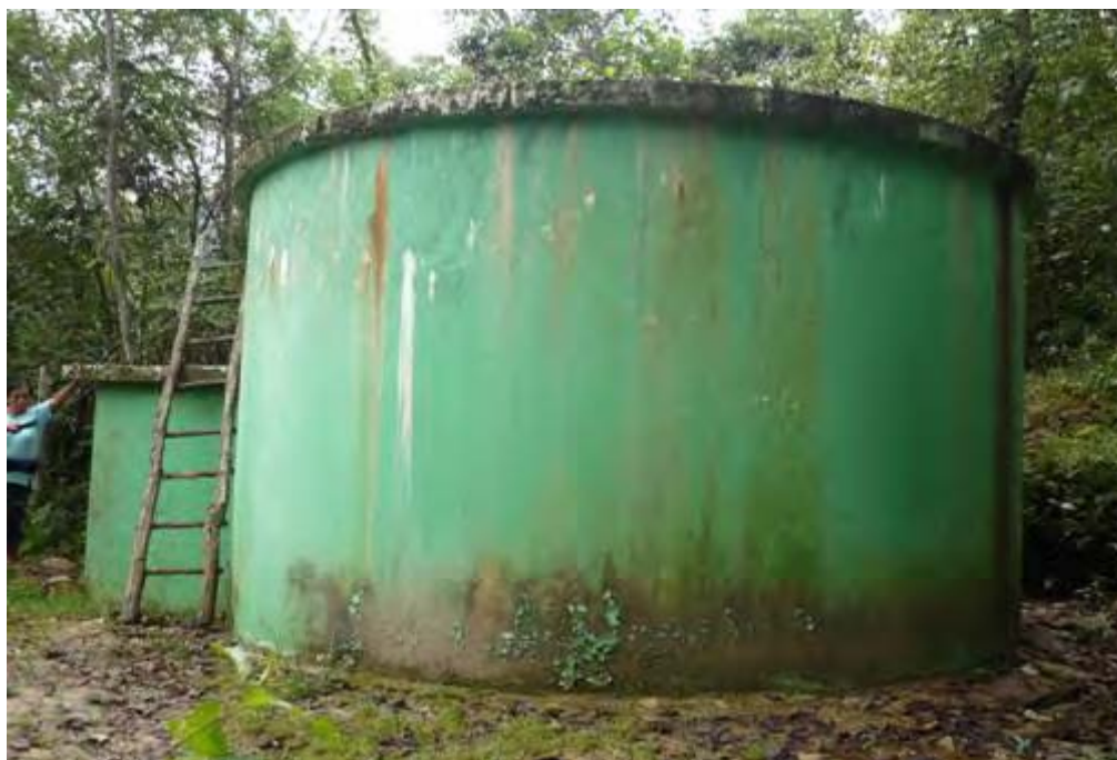
Circular Reservoir - 35 m 3 - San Carlos
