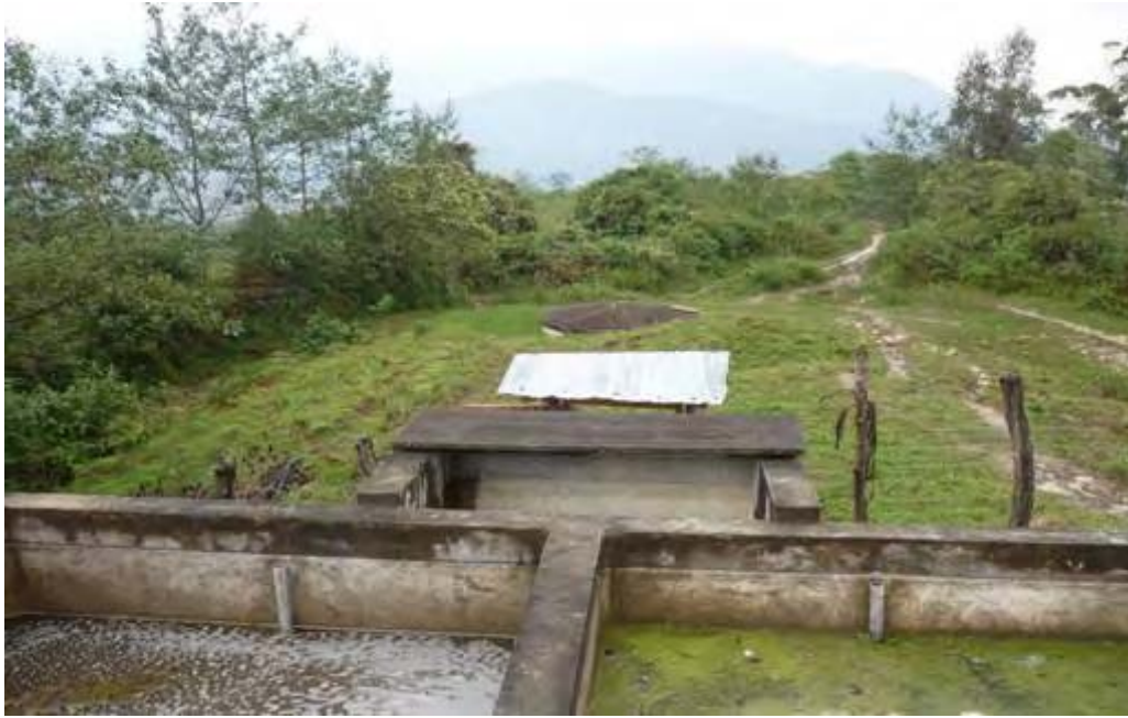
Water treatment – Slow Filters and Reservoir
