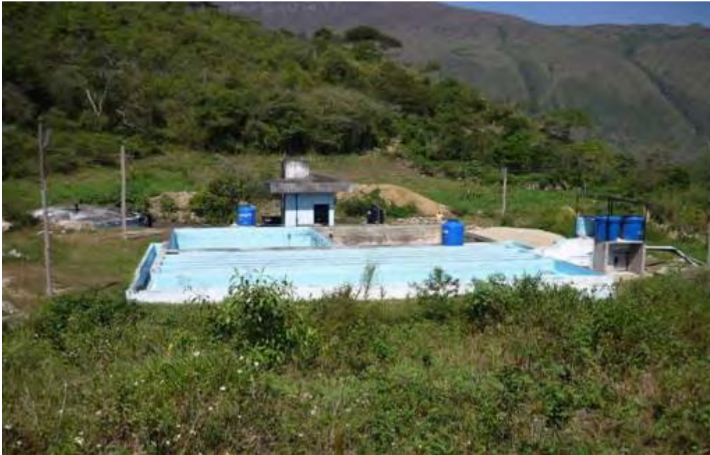
Treatment Plant – Second System
