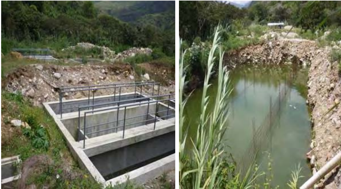
Sewage Treatment - Works
