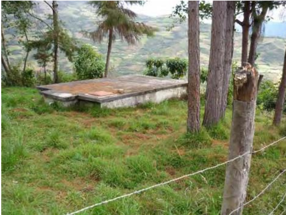
Reservorio V= 25 m 3
