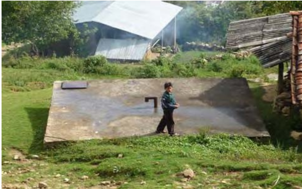
40 m 3 Squared Reservoir - San Pablo
