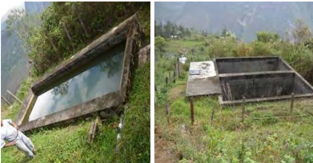
Treatment Plant: Sedimentation tank and Slow Filter - San Pablo
