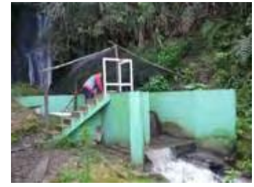
Intake at Ollapata creek in San Carlos
