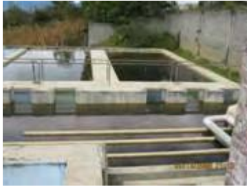
Sewerage Treatment Plant in Lamud
