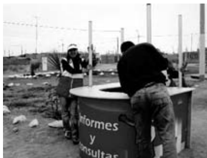
Photo: Technical Team is installing very quickly the Kiosk in the district of la Tinguña Ica, November 2008.
