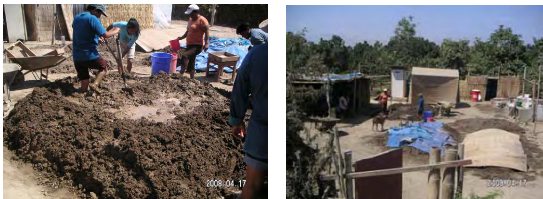
Figure 3.3.2 Training of Reinforcing Adobe House Construction Provided by SENCICO at a Site of Grocio Prado in Cincha Province
