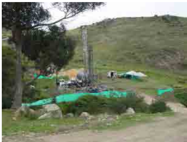
Photo-1 Pilot project site (JICA exploratory well)
