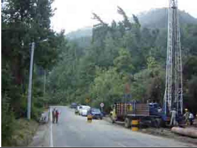
Drilling work by Acueducto in La Aguadora, which is candidate for future pilot project.
