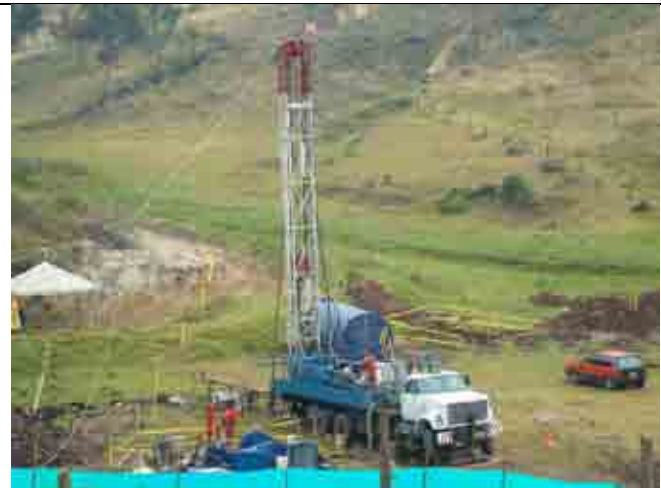
Drilling work by JICA in Ciudad Bolivar, which is candidate for future pilot project.
