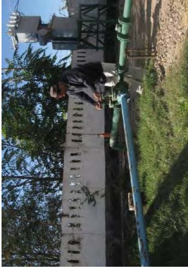
Photo Mé6 Association technician implements water supply adjustment from pump station to the tanks
