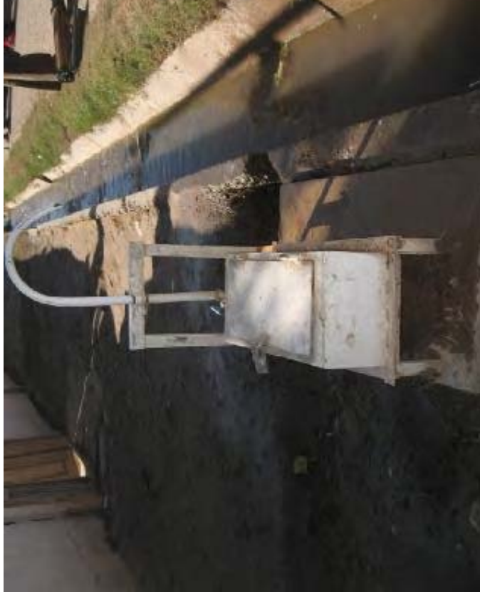
Picture №1-Water supply tap with water meter, of rehabilitated water supply system in Bolshevik village of Qabadiyan district, Khatlon region.
