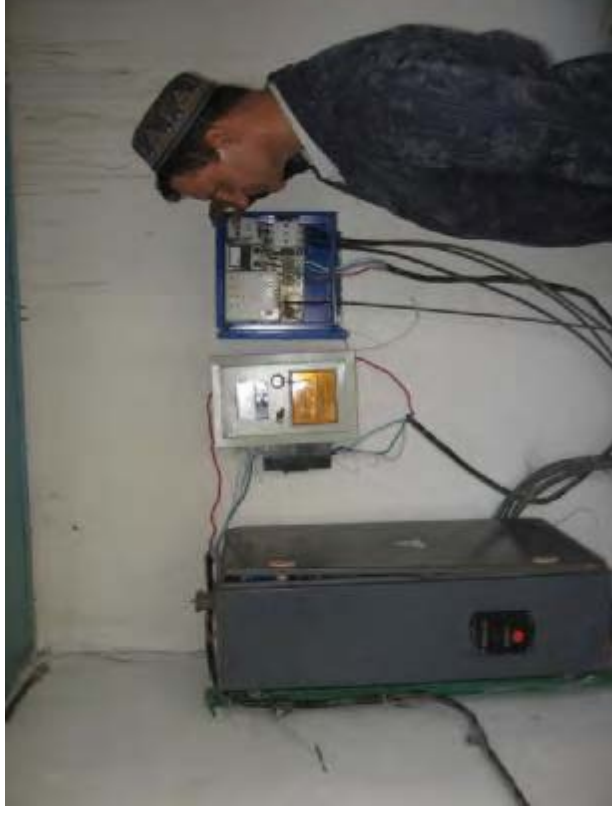
Photo №4. on duty electrician starts the pump.
