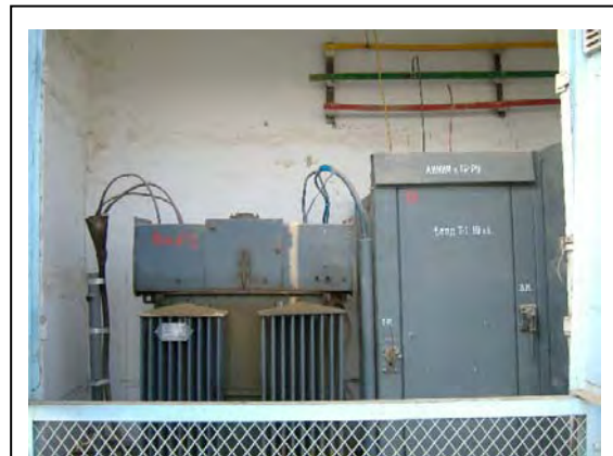
Incoming Panel and Transformer
