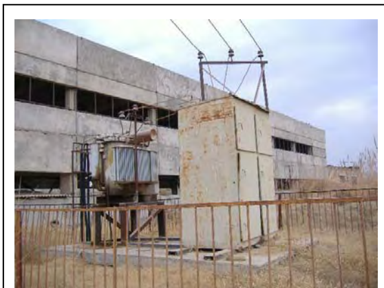
Incoming Panel and Transformer
