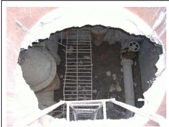
Inside of Vakhsh - Uzun Junction Valve Box
