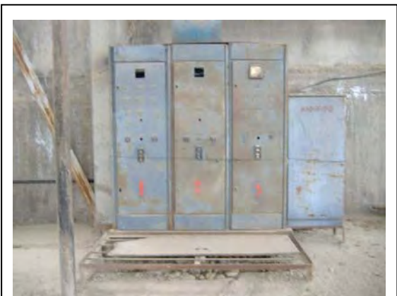
Control Panel for Pump
