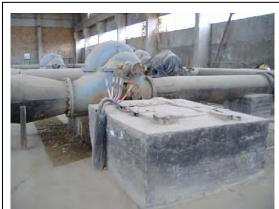
Bokhtar Head Pumping Station
