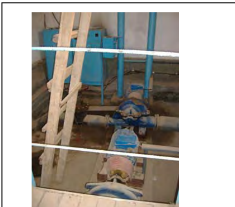
Intake water pumping station 1
