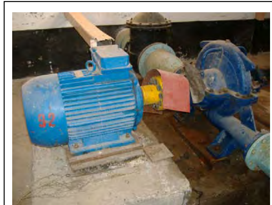
A Pump at New pumping station
