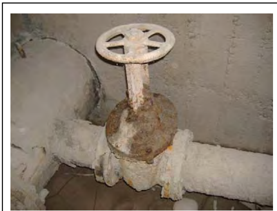
Wash Out Valve inside of Valve Box
