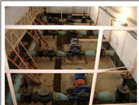
Kalinin New Pumping Station
