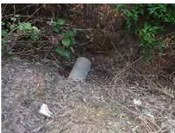
Drainage pipe for treated water
