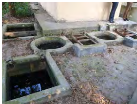
Tanks for chemical treatment
