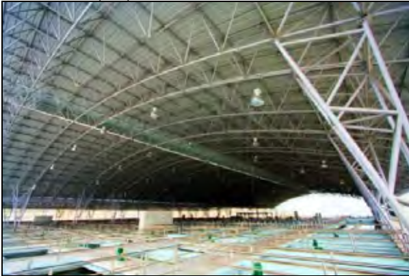
Photo 7: Da River Water Supply Project Main Treatment Process Structure with roof for all process
