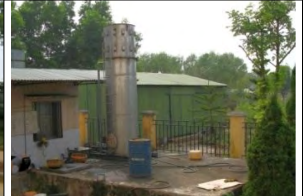
Photo 12: HHTTP Temporary Water Supply System Intake well with compact treatment system at Start-Up Center
