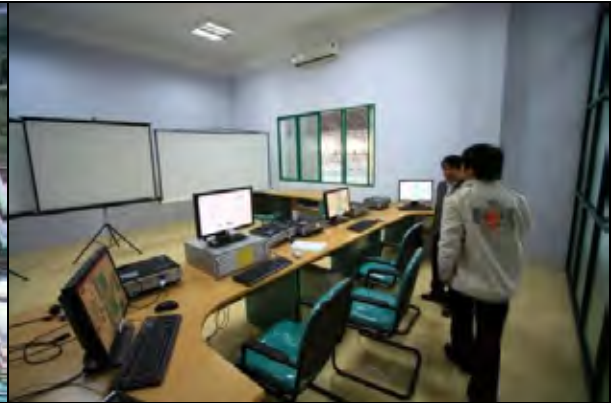
Photo 8: Da River Water Supply Project Main Control Room with all atomized system
