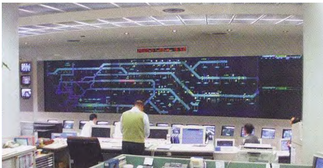
Figure 9.2-2 Example of Traffic Control Center in Japan
