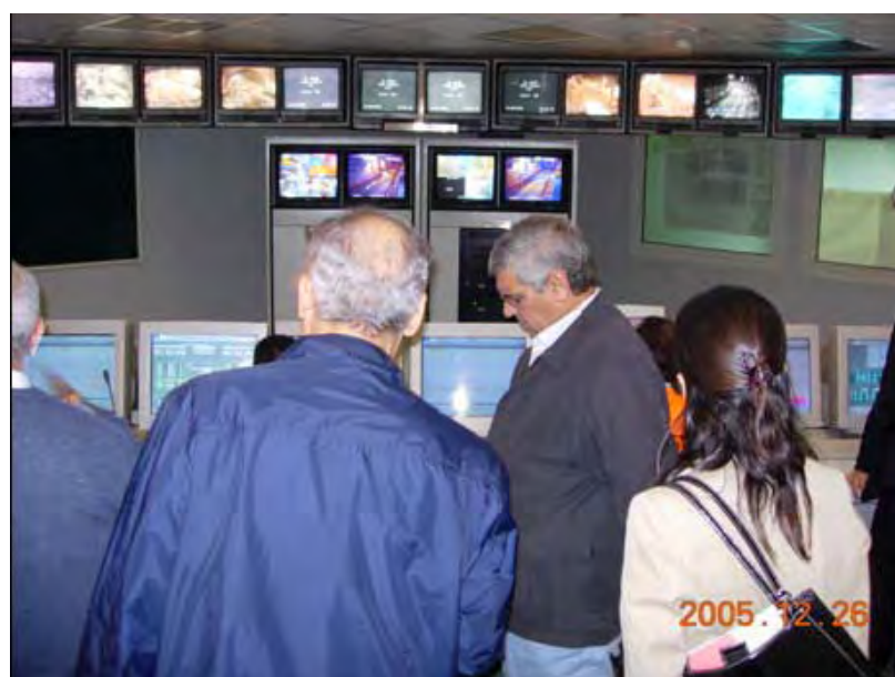
Figure 9.2-3 Traffic Control Center of Al-Azhar Tunnel
