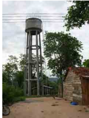
<P-6 Ea Cha Rang> Elevated tank
