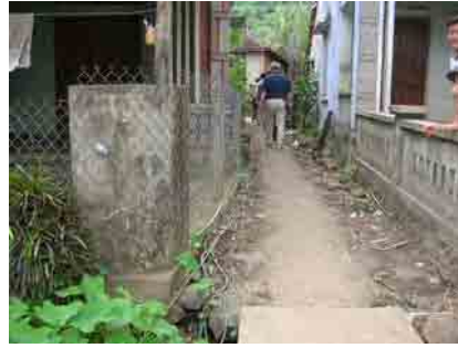
<P-3 An Tho> Distribution pipe
