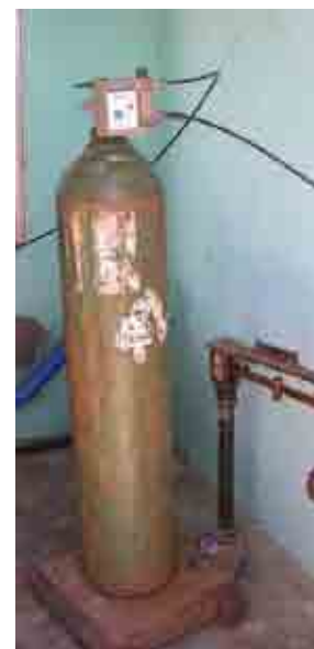
Small type gas chlorinator (Binh Thuan province)
