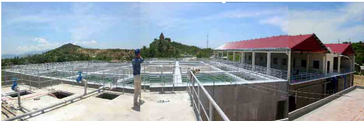
Thap Cham water treatment plant in Ninh Thuan (capacity: 20,000m 3 /d)
