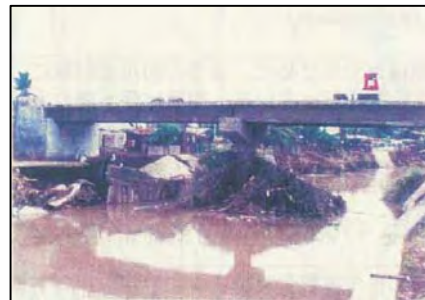
Photo- 2 Debris under Bridge after the Flood of Typhoon Reming Oct 2000 (Source: IDI-Japan)
