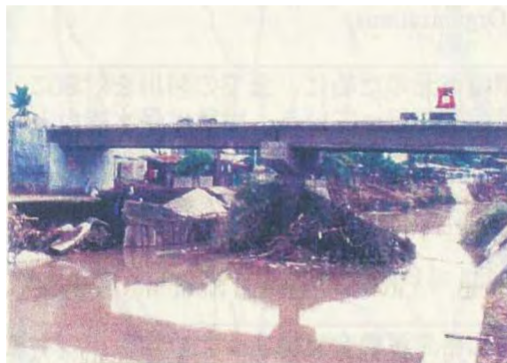
Fig. R 5.6 Clogged Bridge (Ylang-Ylang Bridge)
