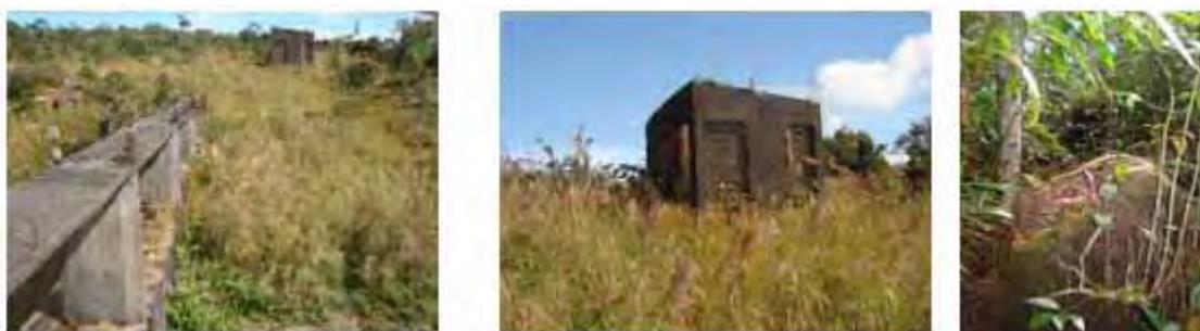
Photo 3-4: Damaged water intake (left), pump house (centre), water pipeline support pier (right)
