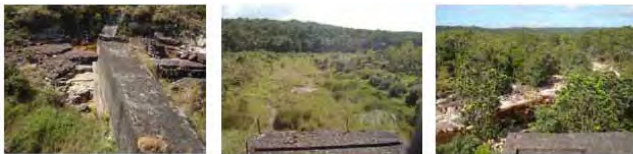
Photo 3-3: Damaged water intake (left), hill where this small river begins (centre), downstream flow to Bokor project site (right)
