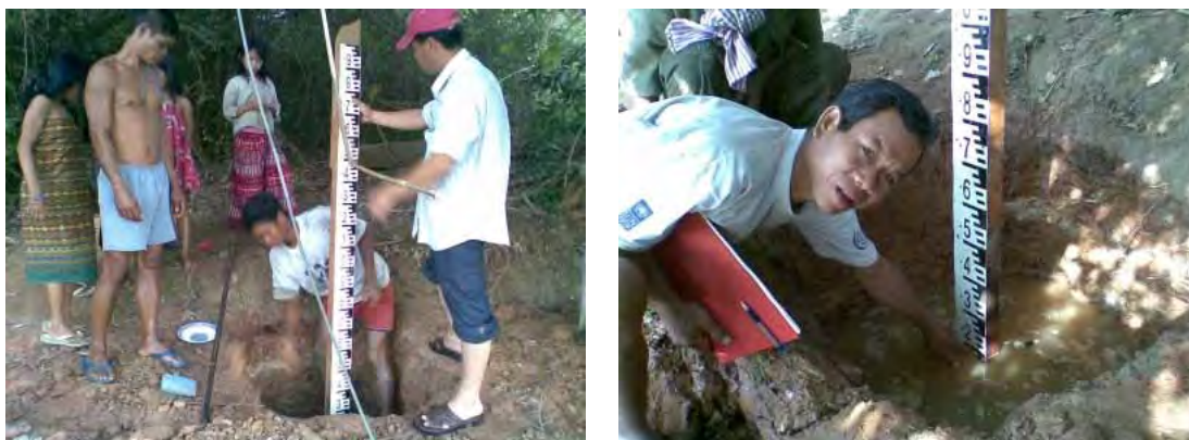
Installation of staff gauge in Yon Village, on the right bank of the Prek Liang River
