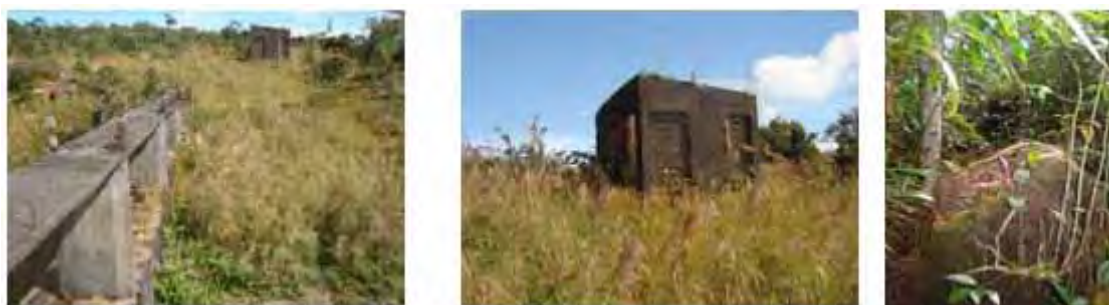
Photo 3-4: Damaged water intake (left), pump house (centre), water pipeline support pier (right)
