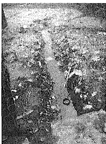
Photograph 7 Drainage in rural market (Bagerhat District)
