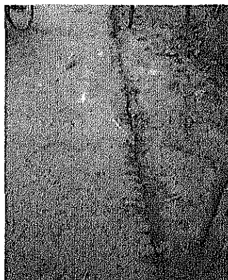
Photograph 1-2 End edging and soft shoulder of Upazila road (Bhola District)
