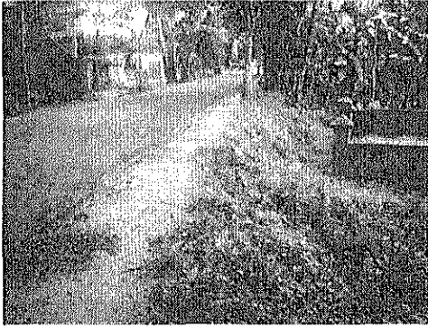
Photograph 1-3 Soft shoulder on Upazila road (Barguna District)
