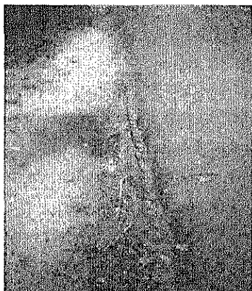
Photograph 1-1 End edging and soft shoulder of Upazila road (Barguna District)
