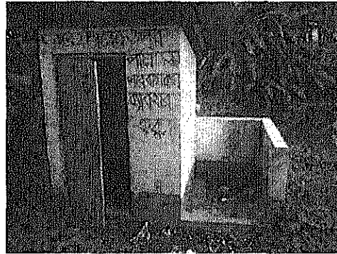
Photograph 4 Unsanitary toilet facility (Khulna District)
