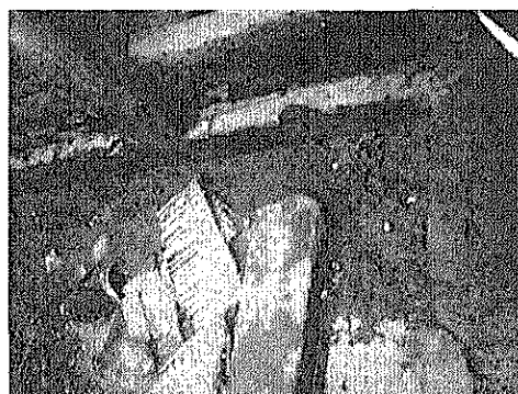
Photograph 8 Drainage in growth center (Bagerhat District)
