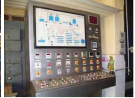
Centralized control panel of Parwanoo plant
